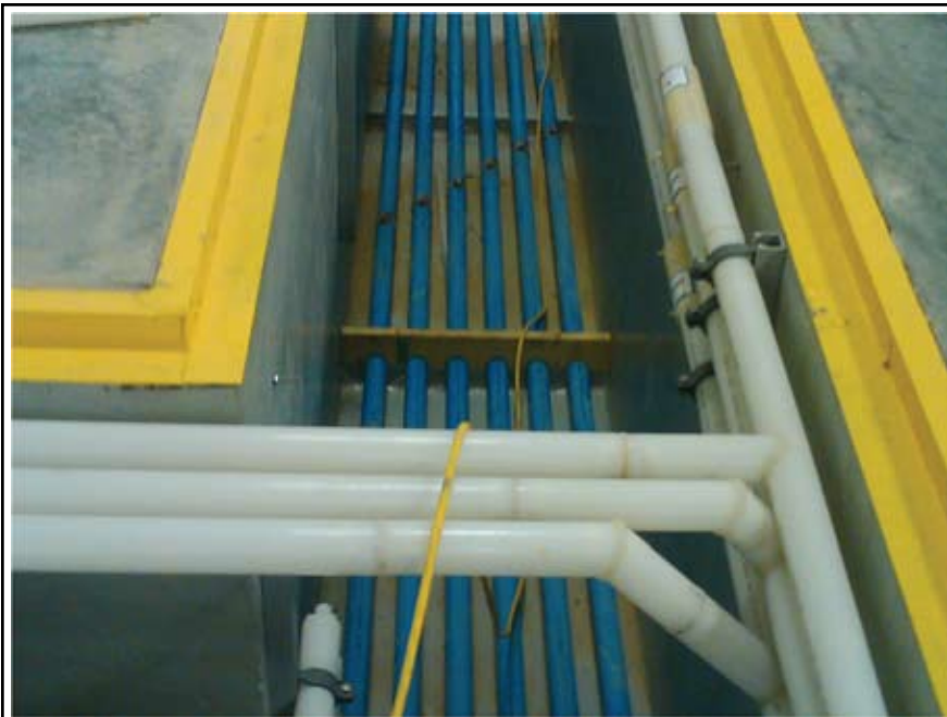
Figure 5. Example of ASTM E84 (25/50) compliant pipe in a construction floor space.
