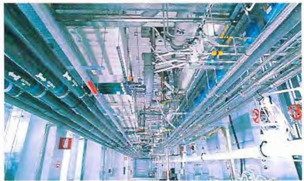
KYNAR PVDF pipes at SGS-Thomson Microelectronics' laboratory in Agrate Brianza, Italy, preserve purity.
