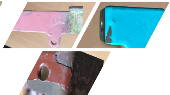
POOR MASKING WITH EPOXY COATINGS
